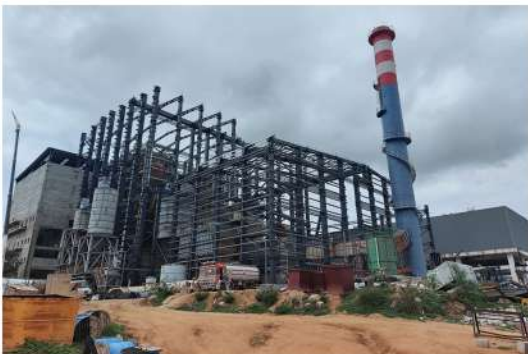
WASTE TO ENERGY PLANT
